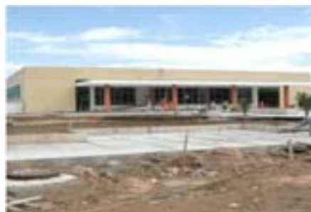
Fig. 1: One of the University Canteens being build on Federal University of Rio de Janeiro (UFRJ) Campus. (Credit: UFRJ Imagens - Marcella Martha)
