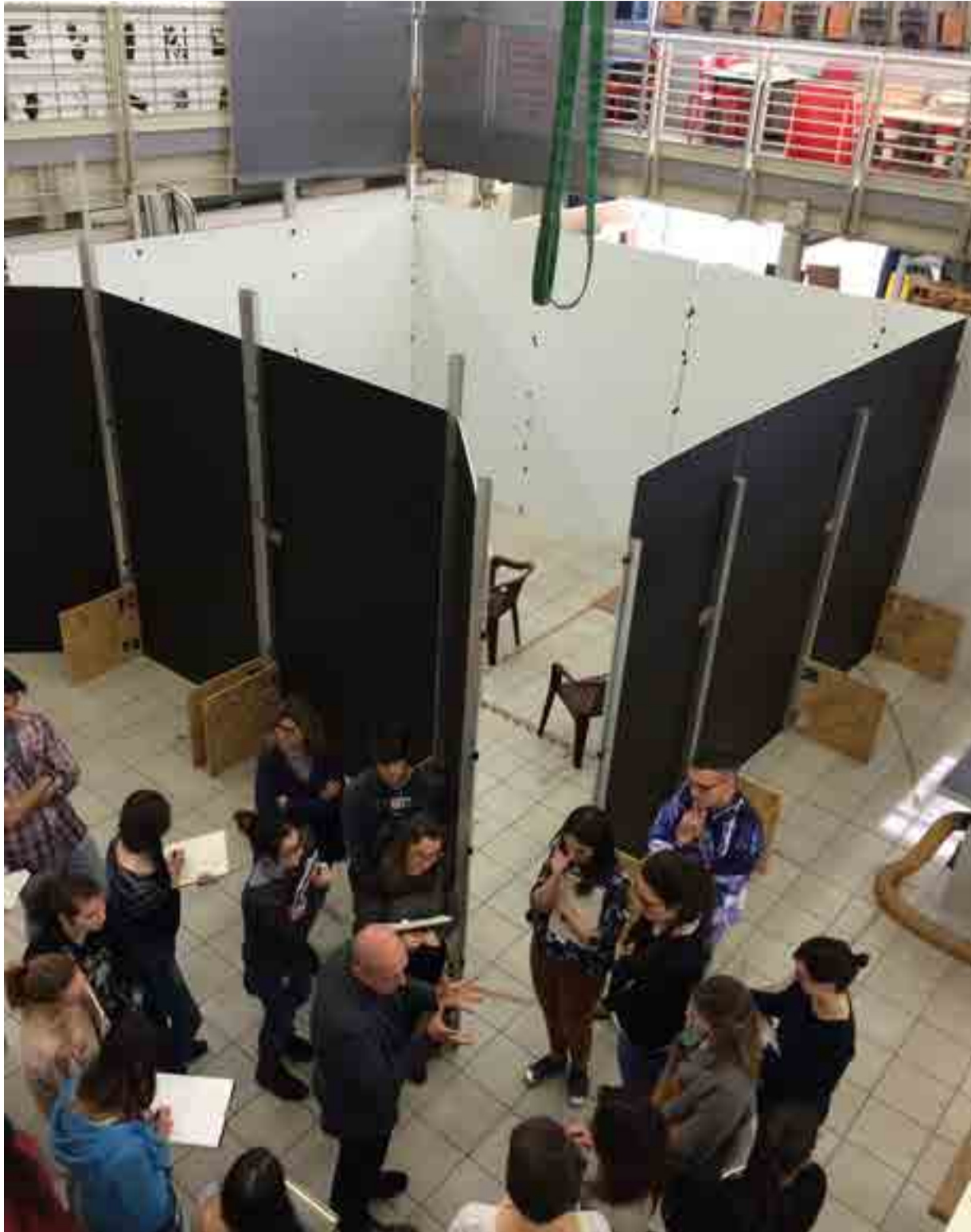
Fig 25.1 Step (a): building a mock-up of a 20 m 2 square room. Personal photograph by author. 2017.
